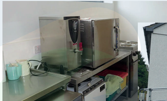
New kitchen equipment
